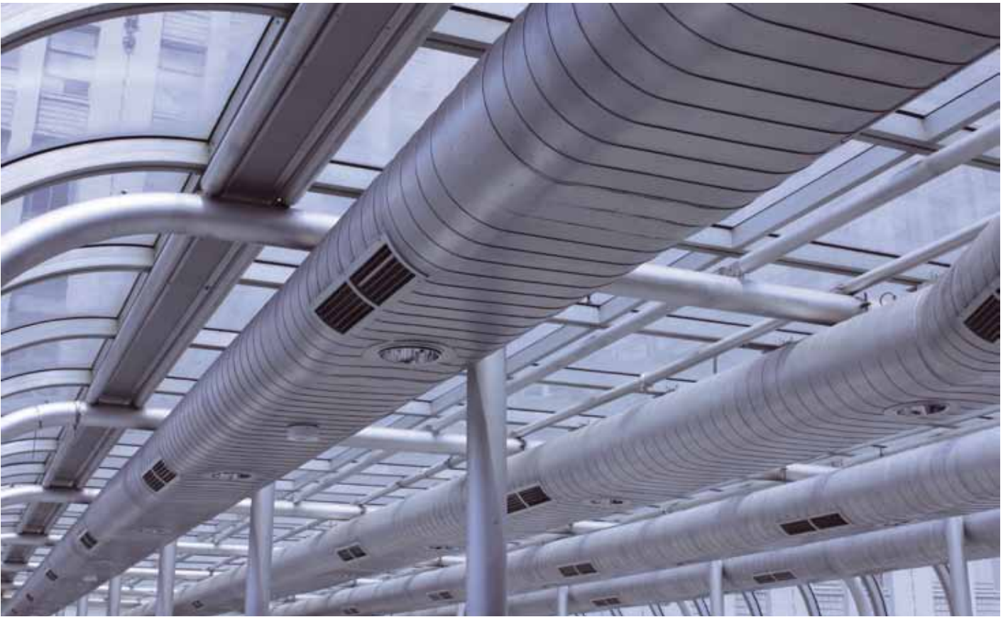
R717 – used in large air conditioning systems (chillers).
