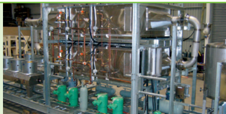
Ethylene-propylene cascade system used for recovery of petrol vapour at -80^{\circ}\text{C} . It uses hermetic compressors (green items visible at the edge of the unit)
