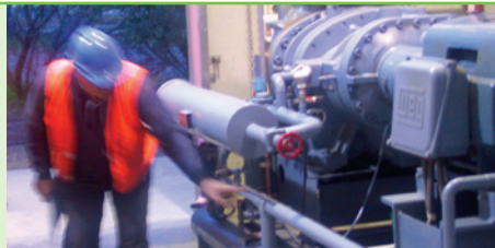
Plant room of an ammonia refrigeration plant room at a cold storage facility in Victoria
