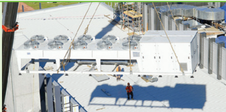
GEA Grasso ammonia chiller being installed on a building roof in Sydney
