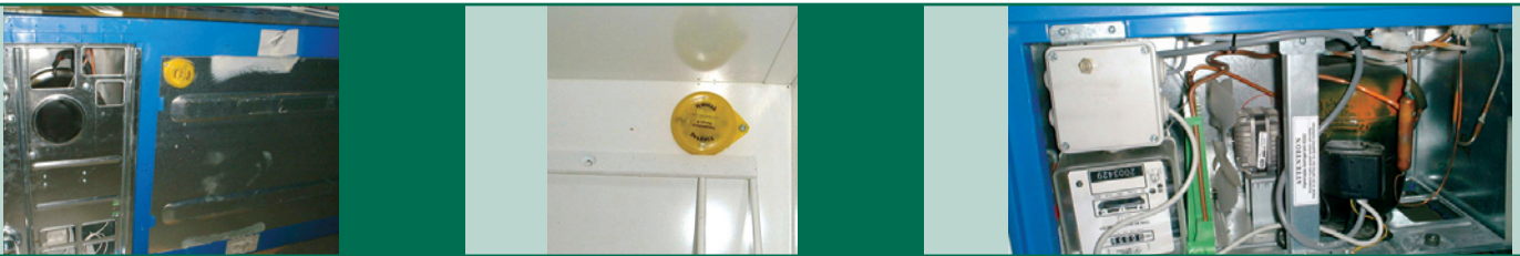
(L-R) Data loggers inside and outside the Unilever ice cream cabinets, and an electricity meter placed on the bottom of the cabinets
