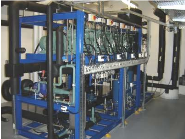
NH 3 glycol Chiller
