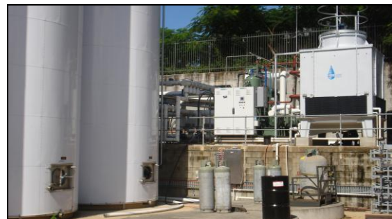
Installed System at Sirromet Wine
