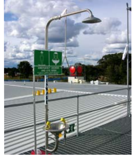
Rooftop emergency shower and eyewash facility
