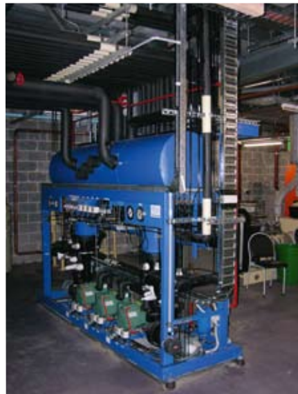
Inside the carbon dioxide system plant room
