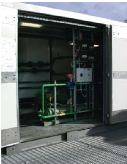
Contained rooftop ammonia plant room
