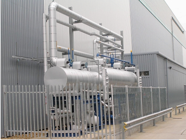
Star Refrigeration's LT & HT surge drum packages
