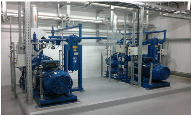
Compressor plant room
