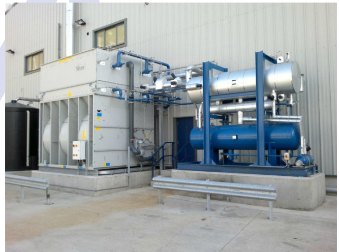
Evaporative condenser connected to the combined surge drum and high pressure receiver package unit
