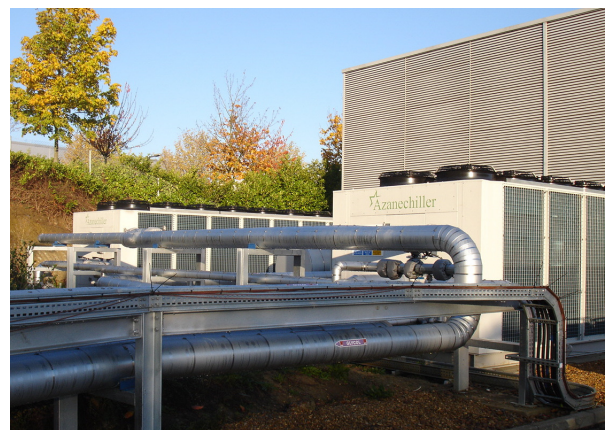
Star's Azanechiller at Kuehne+Nagel, Brinklow
