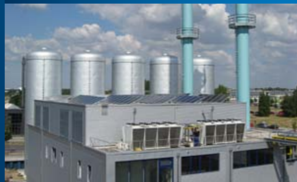
Energy and process cooling
