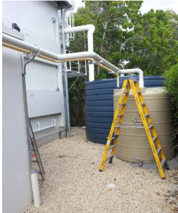
Figure 9. Rain Water Storage Tank for Evaporative Condenser Make-Up Water
