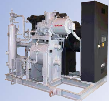
NH3 / CO2 Secondary Cooling Systems
