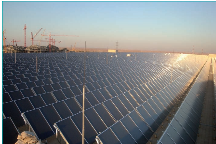
Figure 14 - The world's largest district heating plant with 25MWth installed capacity (36.000 m 2 ) in Riyadh is equipped with European collector technology. (Source: AEE INTEC)
