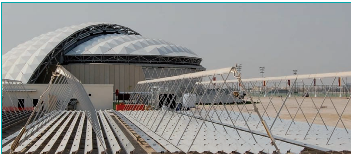
Figure 21 - Solar cooling system with Fresnel concentrator collectors for the showcase football stadium in Doha, Qatar. Source: Industrial Solar
