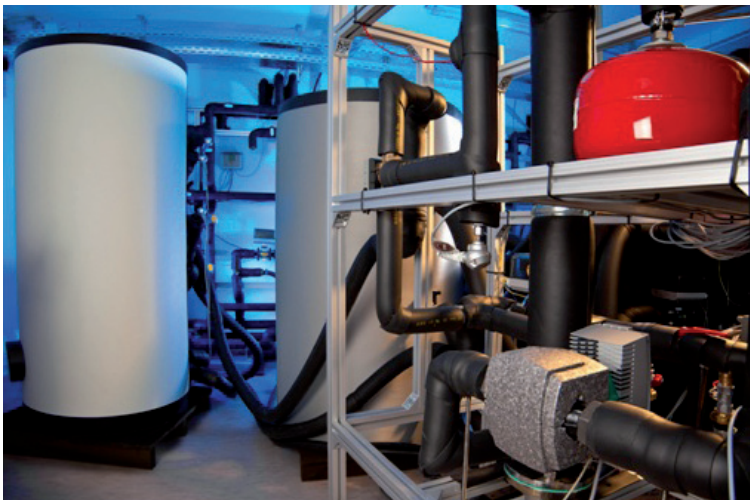
Figure 31 - Water storage test rig. Source: Fraunhofer ISE
