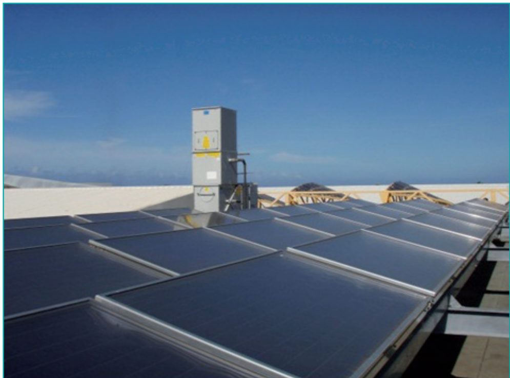
Figure 20 - Solar collector field and cooling tower of a small solar cooling system. Source: Tecsol
