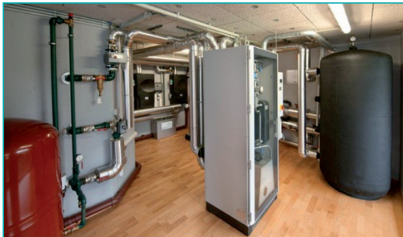
Figure 22 - Absorption chiller of a small solar cooling system. Source: Pink
