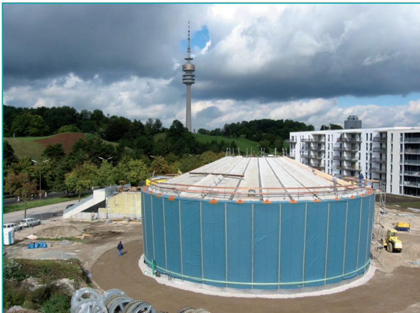
Figure 17 - 6000 m 3 seasonal water storage for a solar district heating system in Munich, Germany, before being completely covered with soil. Source: ZAE
