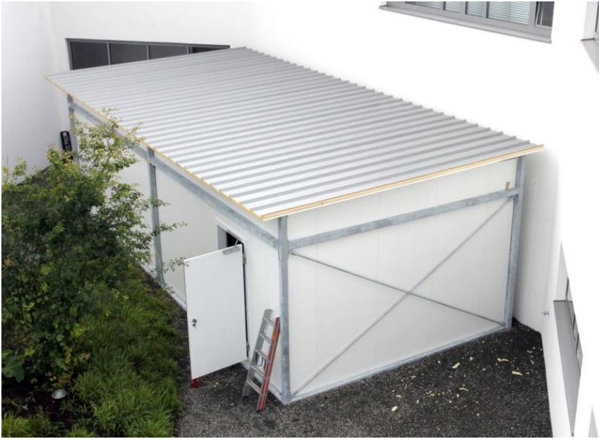
Fig. 5. The cold room in the atrium of the company area of Kramer GmbH in Freiburg-Umkirch (Germany). © Kramer GmbH
